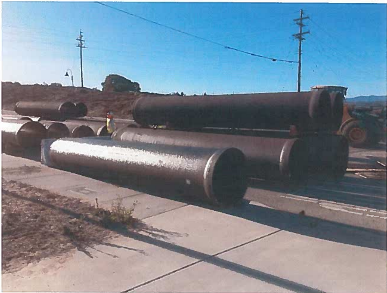
Pieces of a pipeline that was installed by California American Water contractors on General Jim Moore Boulevard. (Monterey Herald file)
